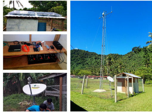
Figure 5: Components of a typical UP CCN installation: solar panels (top left), battery bank and network hardware (middle left), VSAT antenna (bottom left), outdoor GSM radio system, tower and shelter (right).
